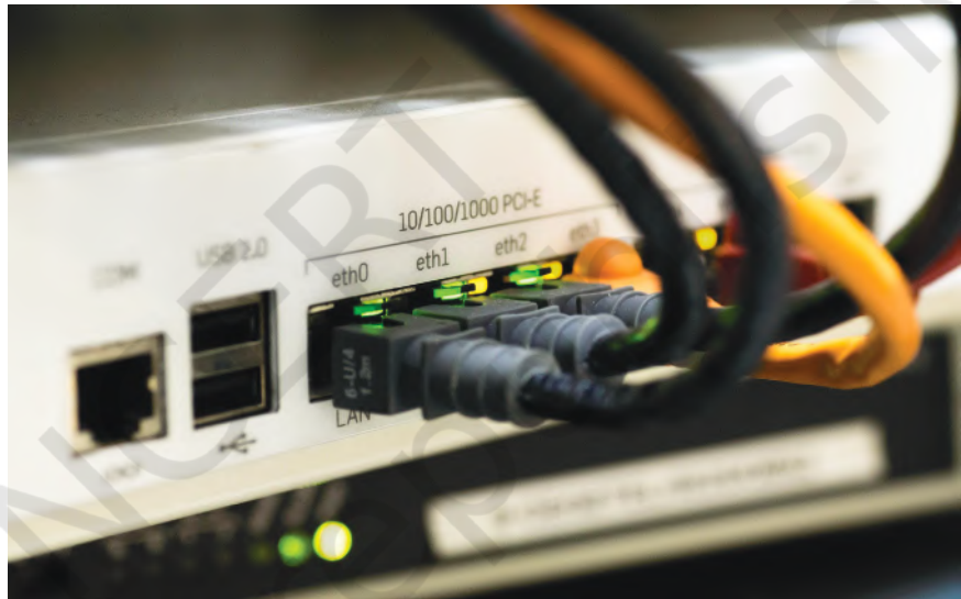
Figure 5.9: Cables connected to a network switch
